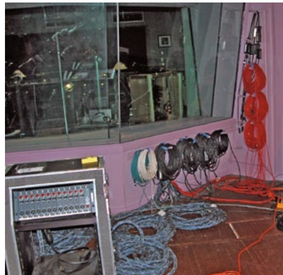
View of the scoring control room from the Scoring Stage. Note the MIT Proline cables at the ready for the next job.
