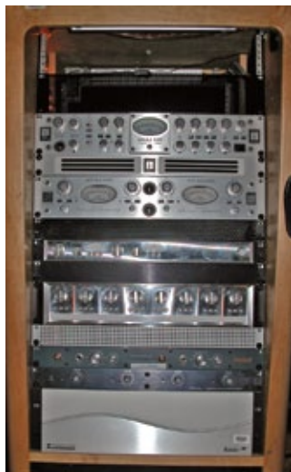
Closeup of one electronics rack inside the Scoring Control Room. There are 2 Z-Stabilizers in use such as the one shown here (bottom component).
